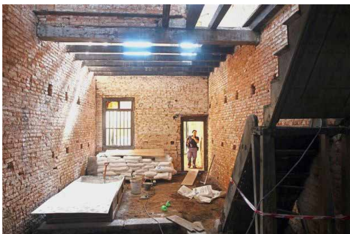
The ongoing restoration work on one of the heritage shophouses in Kimberley Street, George Town.
