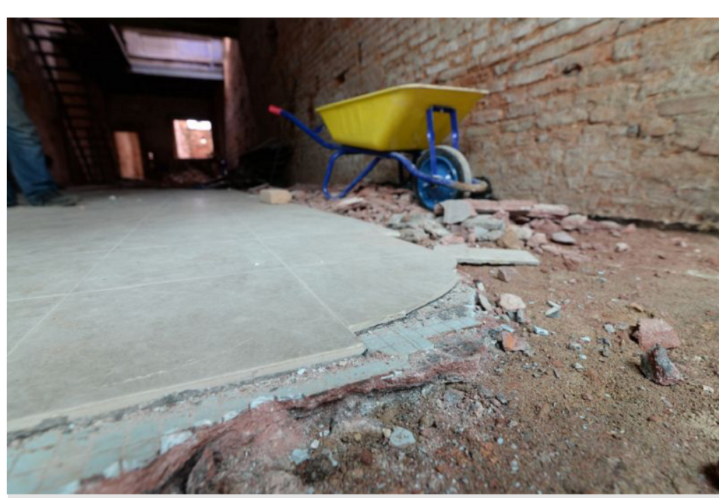
The layers of tiles on the floor tells the history of the pre-war shophouses along Kimberley Street.
