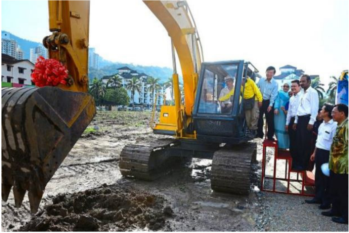
Breaking new ground: Lim at the controls of the excavator during the ceremony at the project site in Relau. — Photo by GARY CHEN
