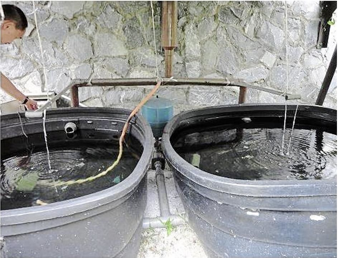
Rainwater harvesting system installed at a community hall as part of MBPJ low carbon framework 2014.
