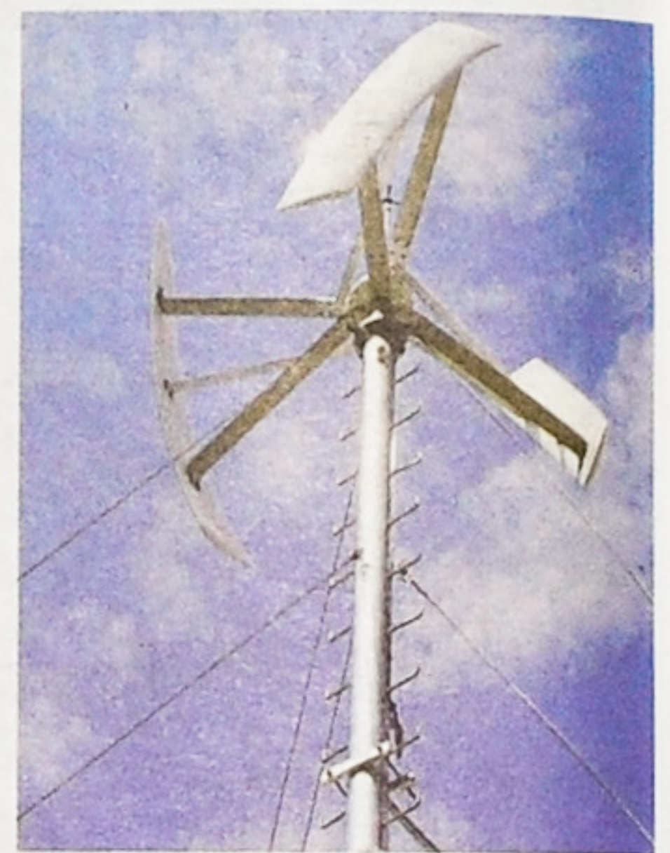
The iWind vertical axis wind turbine in the Instacom compound at the Subang Hi-Tech Industrial Park.
