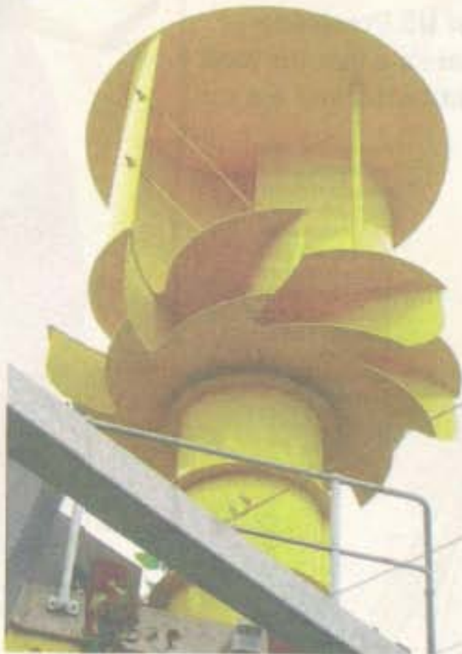
Ventilator turbines on rooftops help harness abundant wind energy in Melbourne. – Dr TAN LOKE MUN
